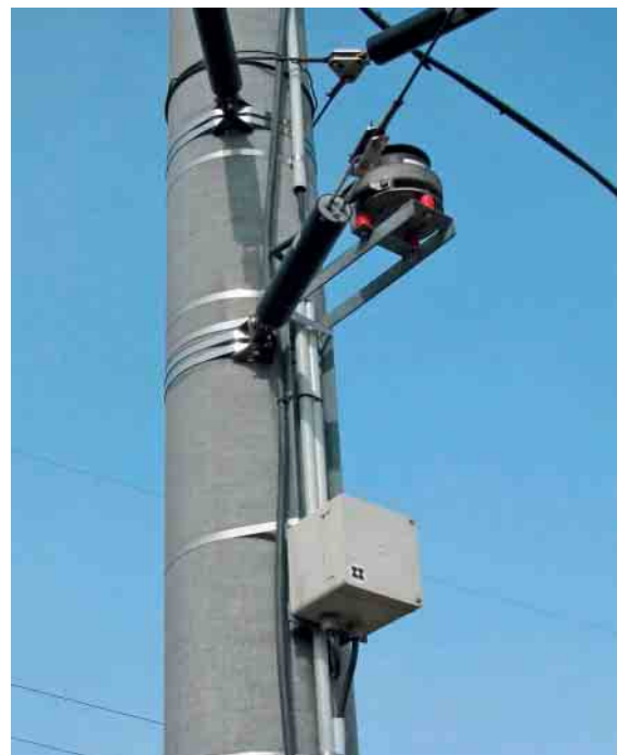
Lightning arrester and pole fuse
