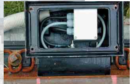
HFK track circuit transformer
