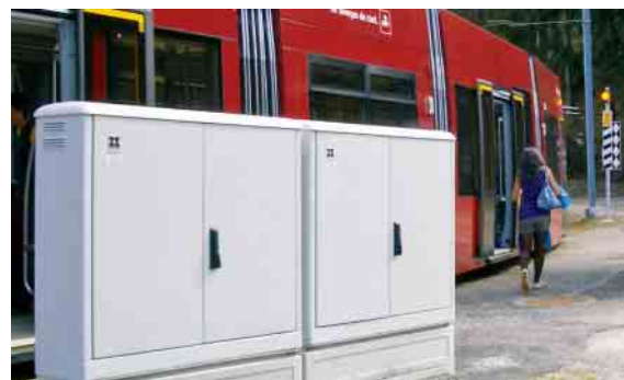
Control cabinets and plinths
